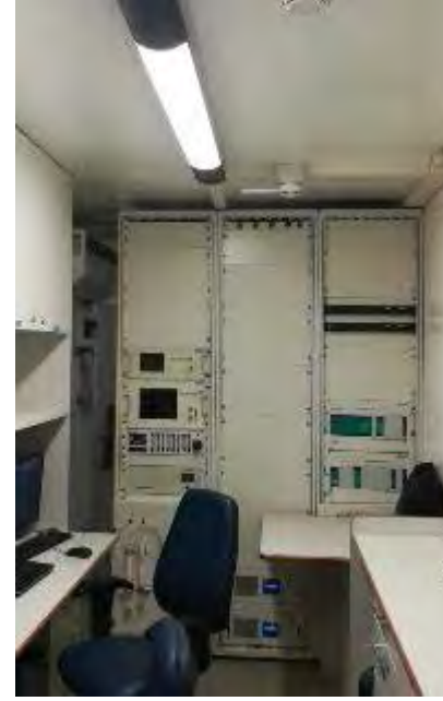
Mud Logging Unit
